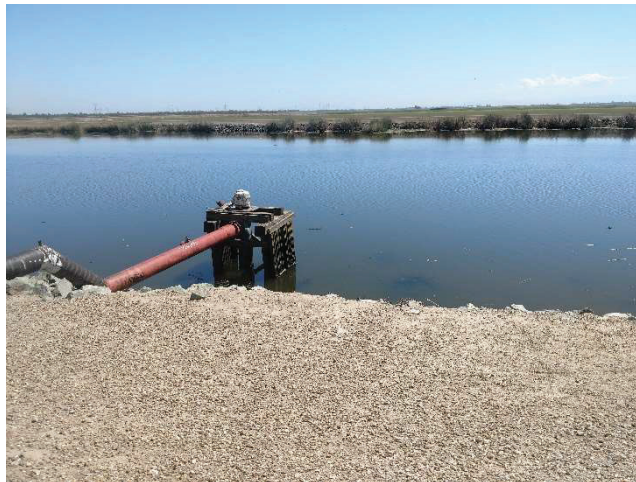
Figure 6 – View of intake pipe on levy adjacent south of subject property, looking south.
