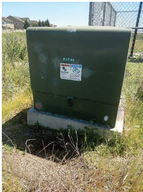
Figure 2 – View of ground transformer, northeast corner of subject property.
